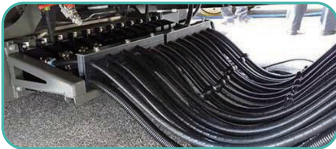
Jumper cables 跳线电缆
