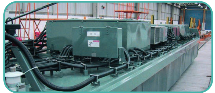
Power distribution 配电
