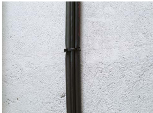
Air conditioning pipes
